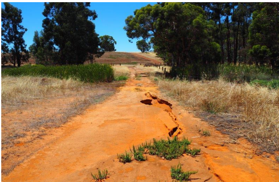
Plate 37. Example of rill erosion on access track at Hotham Farm, January 2017
