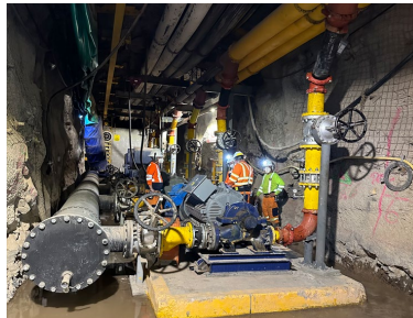
1390L pump station
