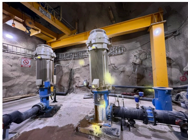
1370L well pumps
